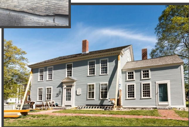
Photo by Janie Dretler taken in June 2016 of Phase I stabilization work in progress.
